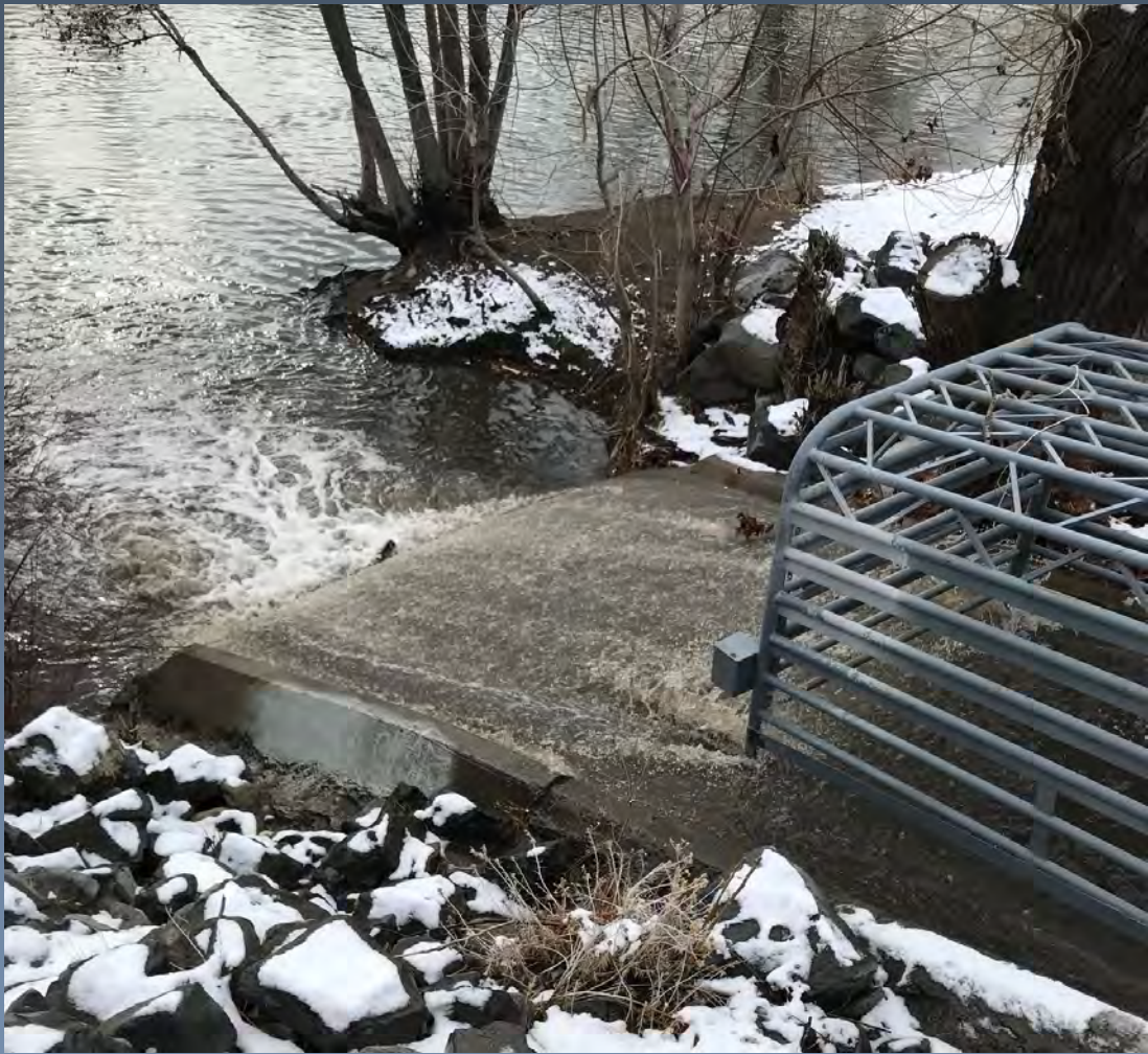
Fisherman's II urban outfall during a storm event
