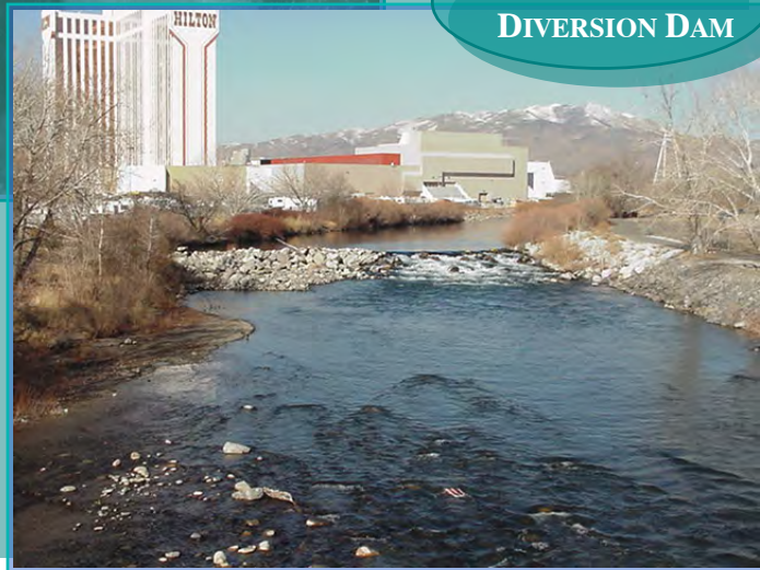
The poorly designed Pioneer Diversion Dam is just upstream of Rock Park.
